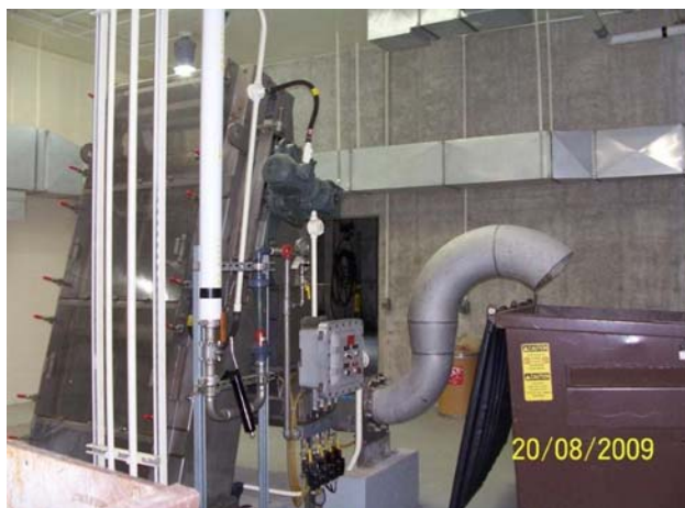
Fine screen removes grease and trash
