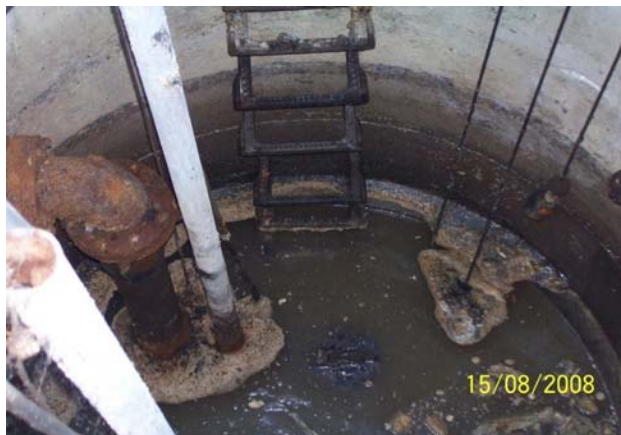
Grease in Lift Station
