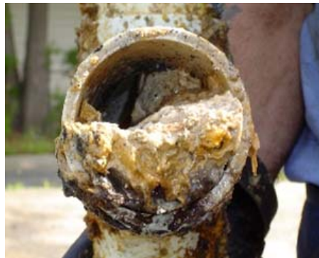
Grease can completely block sewer pipe
